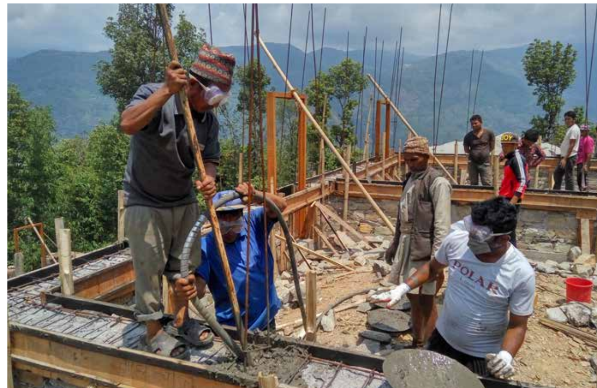
Casting of reinforcement beams in one of the school blocks. The design of new buildings had to be approved by the National Reconstruction Agency.
